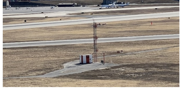
Glide Slope Antenna Serving Runway 4-22
